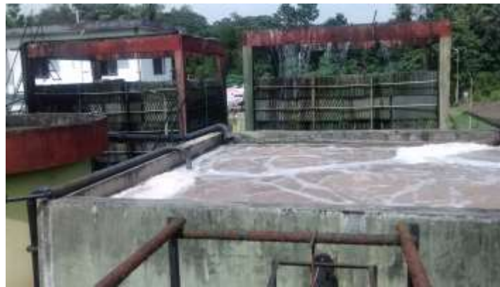
Aeration Tank & Bio Towers
