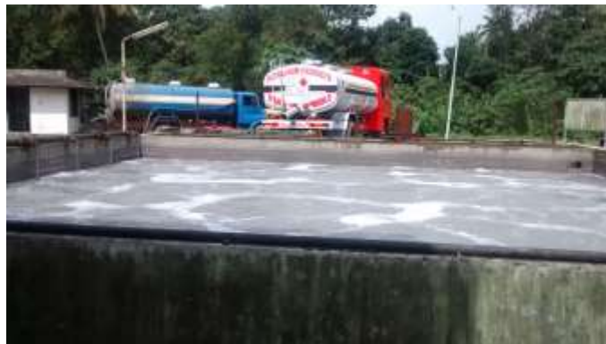
Trucks Carrying Effluent to CETP
