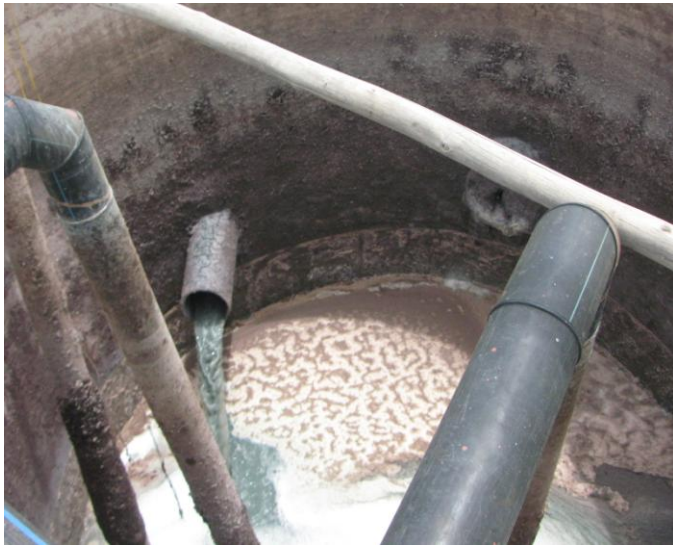
Fig 1: Effluent Receiving tank
