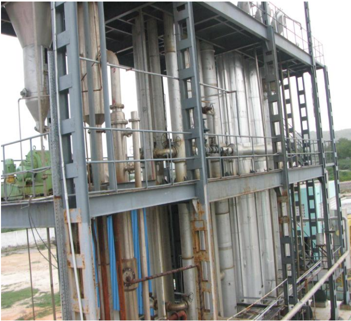
Fig 7: Multi Effective Evaporator
