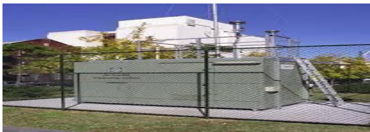
Continuous Ambient Air Quality Monitoring Station (CAAQMS)
