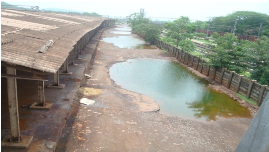
FIGURE 6.5 WATER LOGGING AREA AT SIDING
