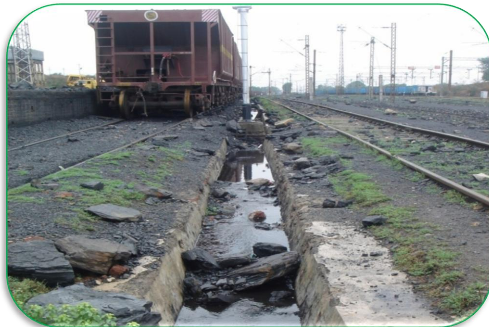
FIGURE 4.16 CHOKED CONDITION OF WASTE WATER COLLECTION SYSTEM
