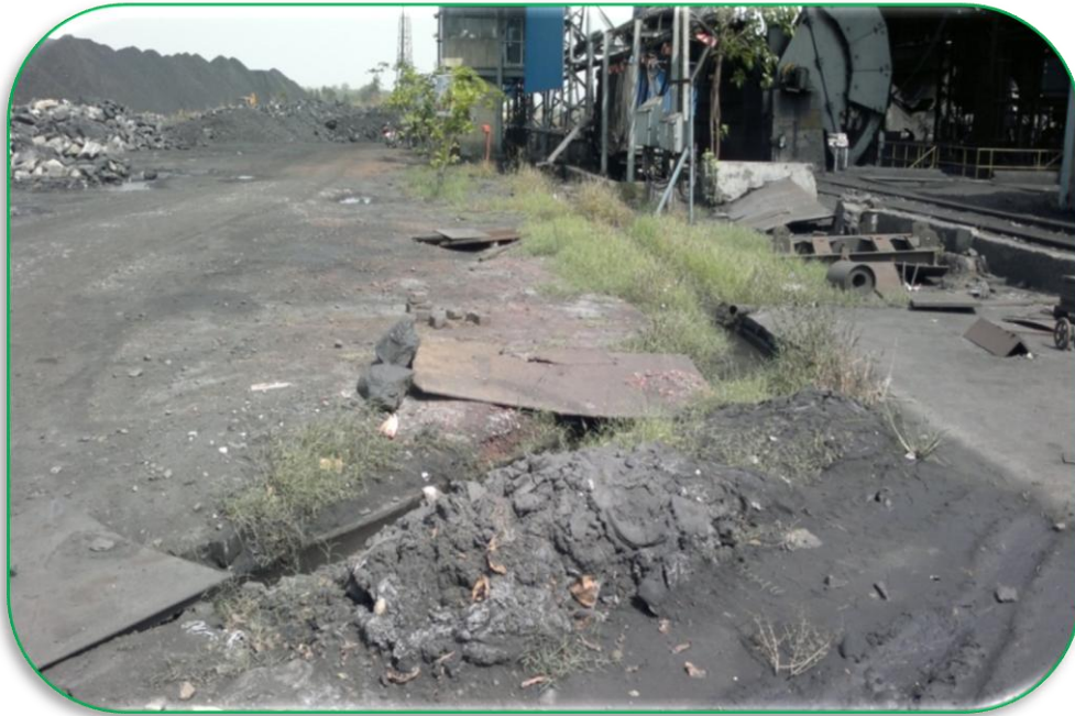
FIGURE 4.15 INADEQUATE WASTE WATER COLLECTION SYSTEM
