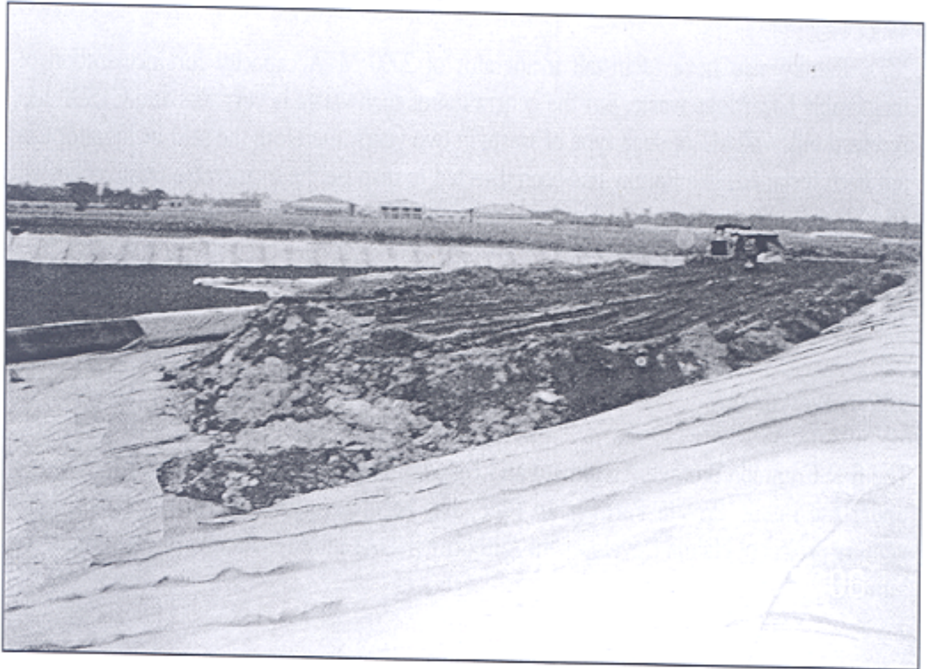
1 st Cell of the Common Land Fill facility at Haldia (In operation)
