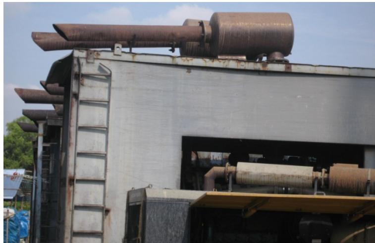
High capacity DG Caterpillar Engines (up to 1250 KVA) are still operated without any acoustic enclosure and the emissions from these engines are released horizontally that too at an inadequate height.
