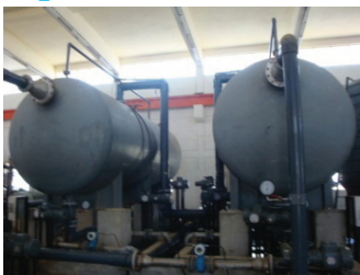
Pressure Sand filter
