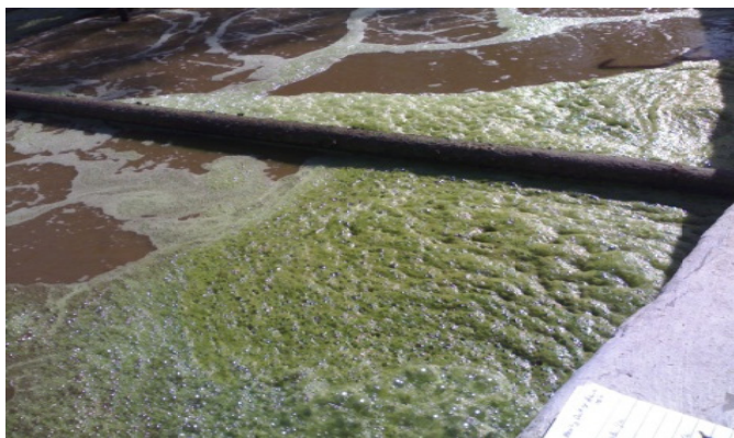
Figure 10.2 : Clarifier-cum-aeration System with Red & Green Algal Growth
