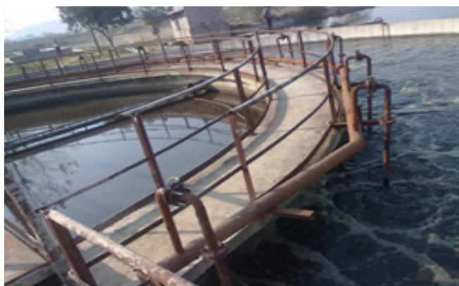
Figure 10.4 : Aeration Treatment Facility
