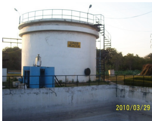
Figure 14.4 : CETP at Govindpura
