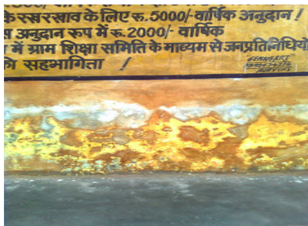
Figure 11.3 : Impact of Chromium leaching on building wall in Rania area, where Chromium rich sludge was used for land-filling
