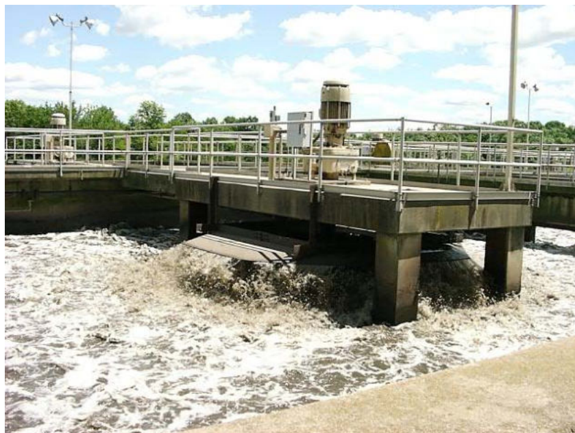
Effluent Treatment Plant
