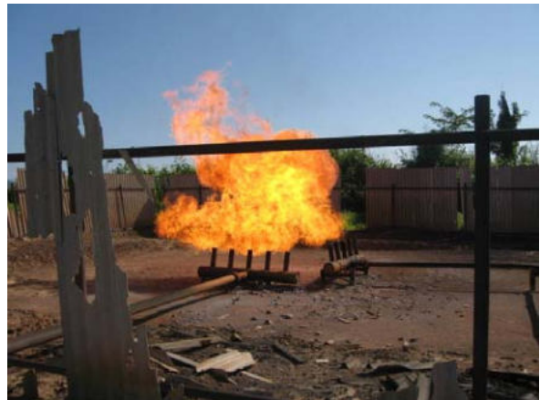
Ground flare without proper enclosure at oil mining site at Arunachal Pradesh
