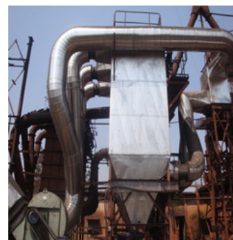
Waste Heat recovery boiler
