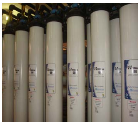
Ultra Filtration Plant of CETP
