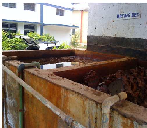
Sludge drying beds of CETP
