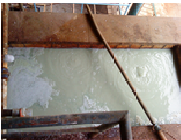
Neutralization tank of CETP
