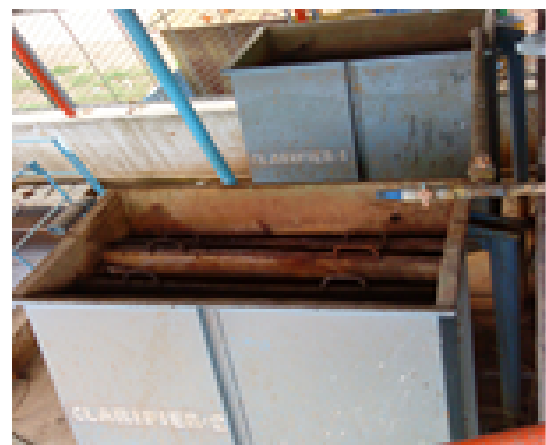
Lamella Clarifiers of CETP
