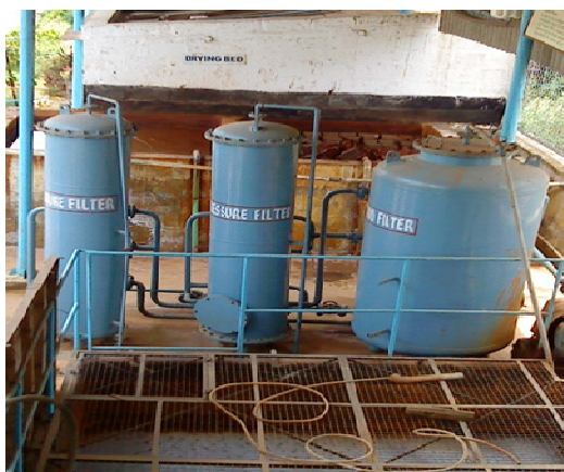
Sand filter and pressure filter of CETP
