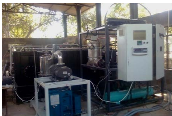
Lyophiliser plant at Kanpur - An actual site view
