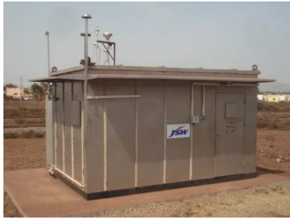
Automatic Air Quality Monitoring Station
