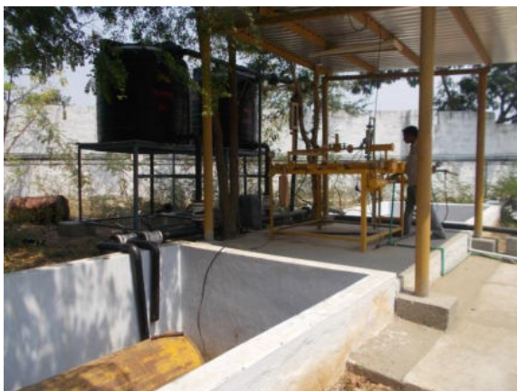
Chlorine gas dosing system to remove colour
