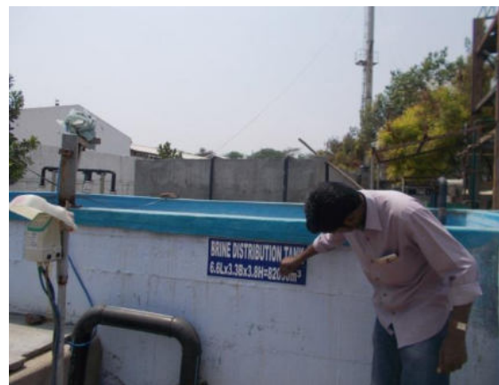
Brine preparation tank
