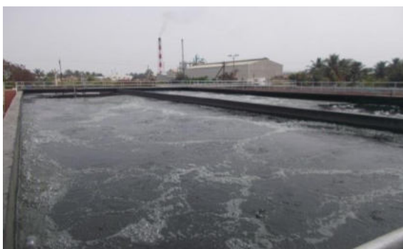
Biological oxidation tank
