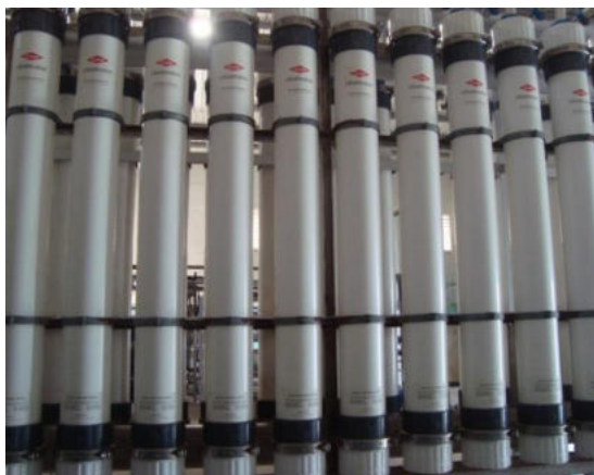
Ultra filtration skid
