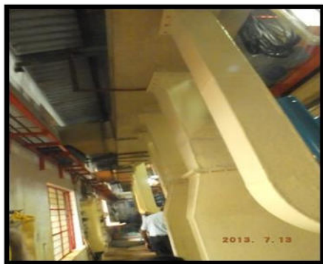
Hood system connected to chimney
