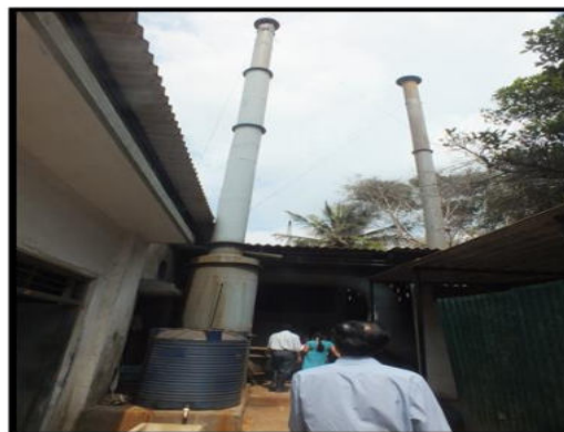
Chimney with water scrubbing system
