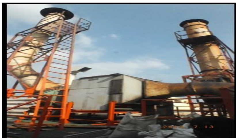
Chimney with water scrubber attached to the hood system.
