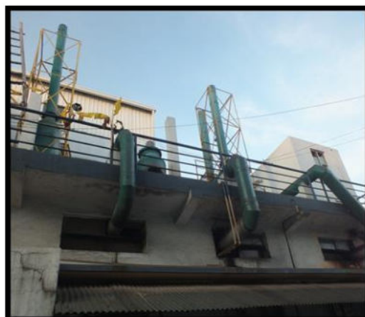
Fume extraction system connected to chimney
