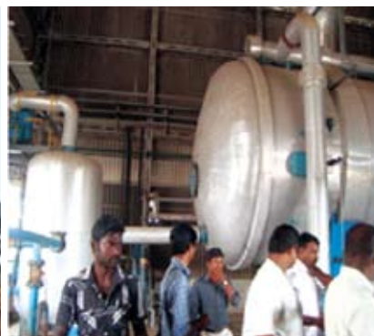
Mechanical Vapour Recompressor
