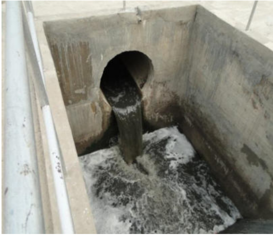
Inlet of STP
