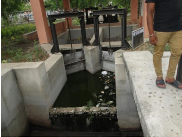
Inlet to STP
