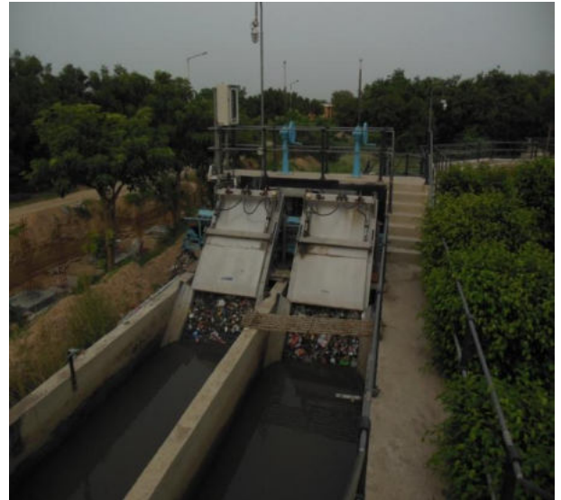
Grit Removal Chamber
