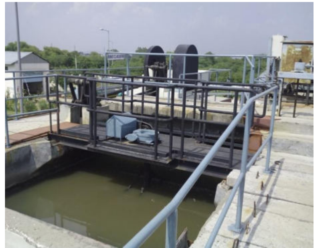
Grit removal system
