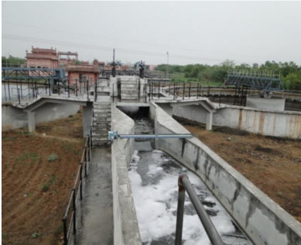
Inlet to STP
