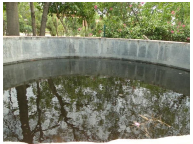
Treated water holding tank
