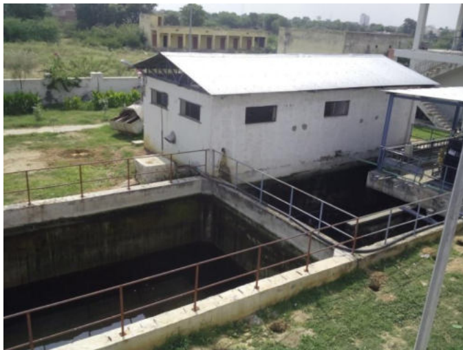
Treated water Collection Tank
