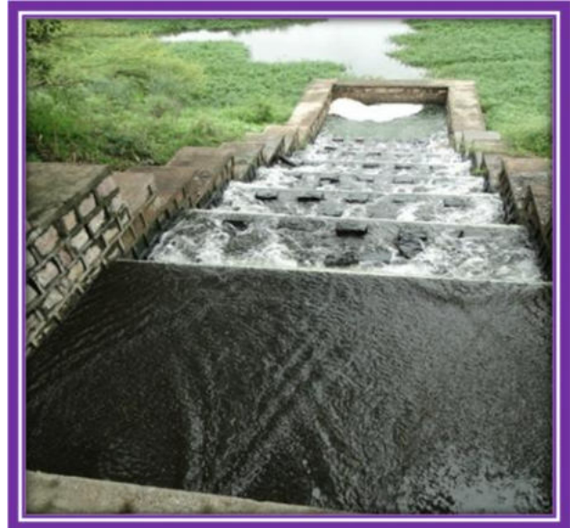
Primary Treatment Unit
