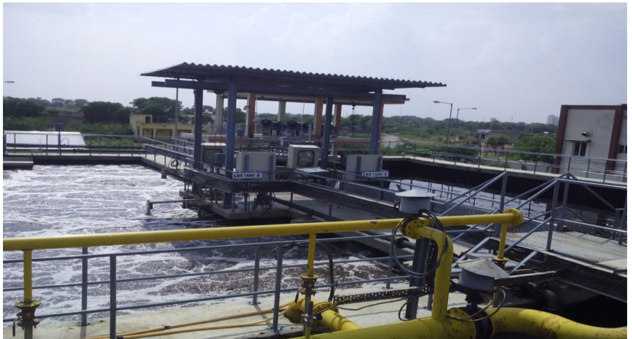
Filtration, aeration, and Nitrification and DO monitoring system
