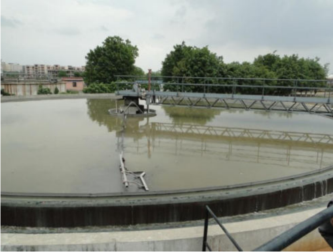
View of the clarifier
