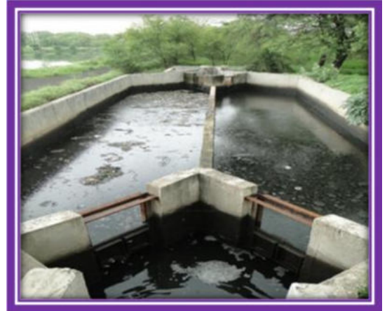
Primary treatment unit
