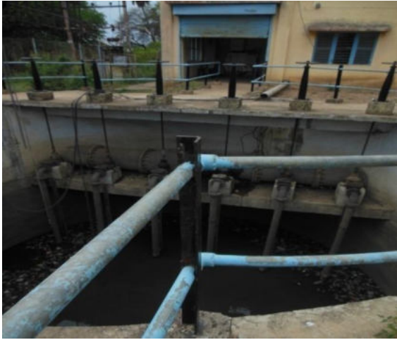
Raw Sewage Collection Tank
