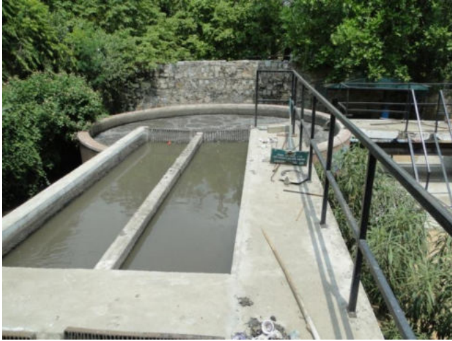
Inlet to STP
