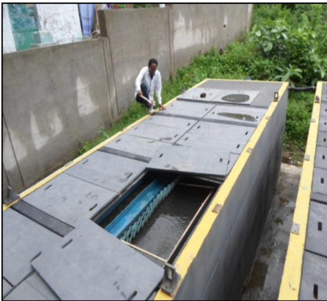
Top view of the fabricated STP
