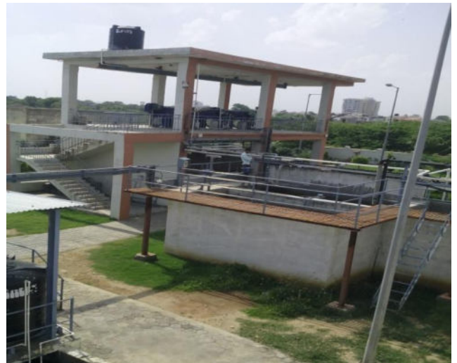
Sludge Sump and Centrifuge Unit
