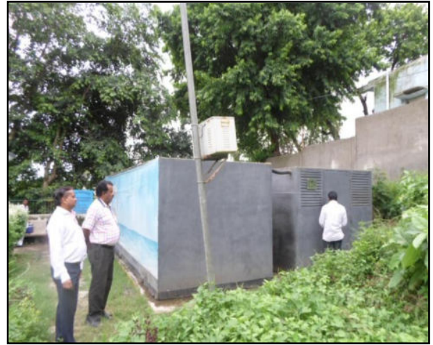
View of the fabricated STP
