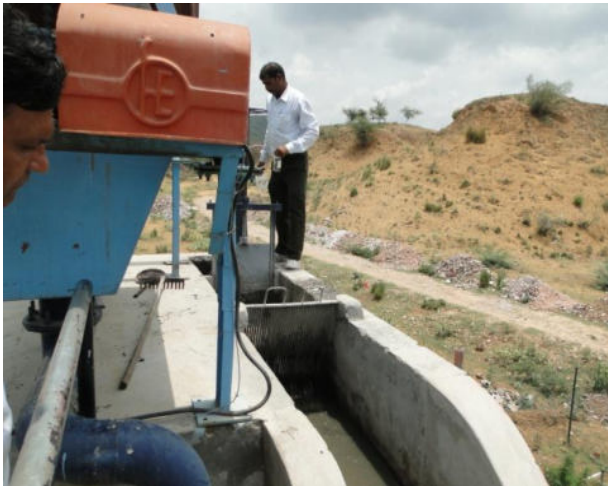
Inlet of STP
