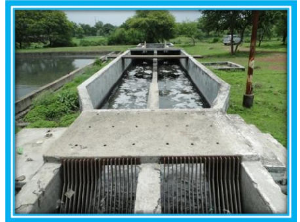
Primary Treatment Unit
