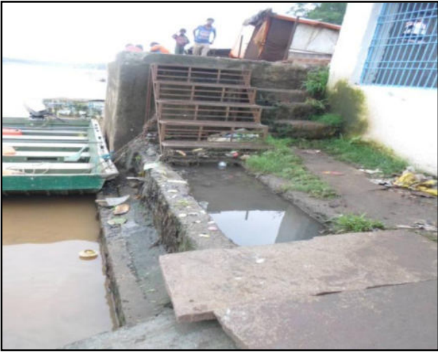
View of the sewage collection pit
