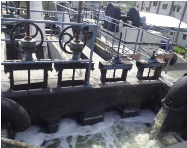
Raw Water Inlet, Fine Screen
