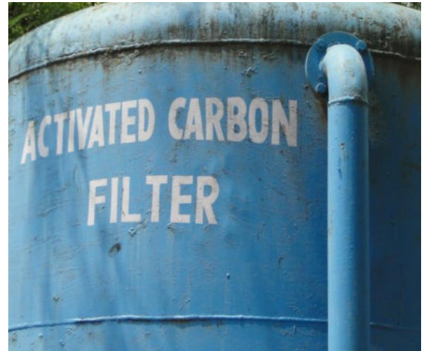
Activated carbon filter
