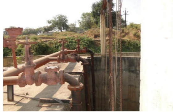
Pumps not being used
