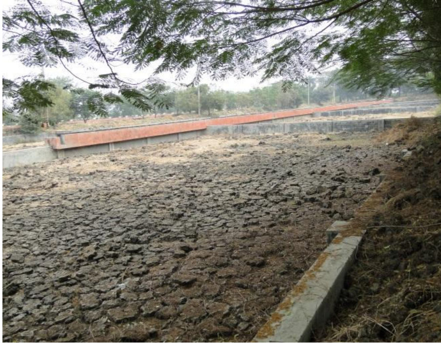
Sludge drying bed
