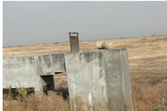
Inlet Channel of Oxidation Pond
