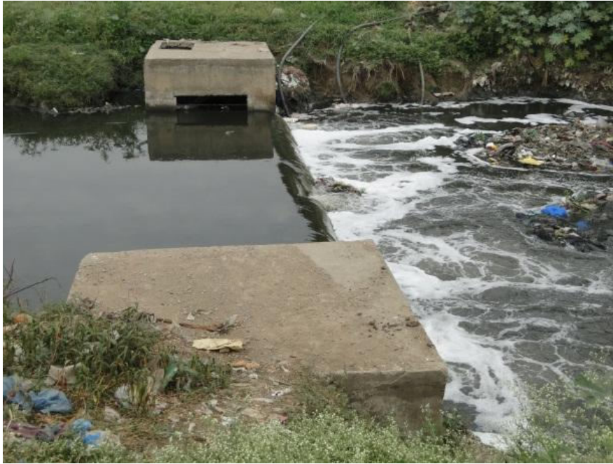
Inlet of STP
