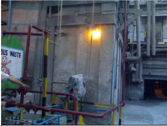
HW pumping system
