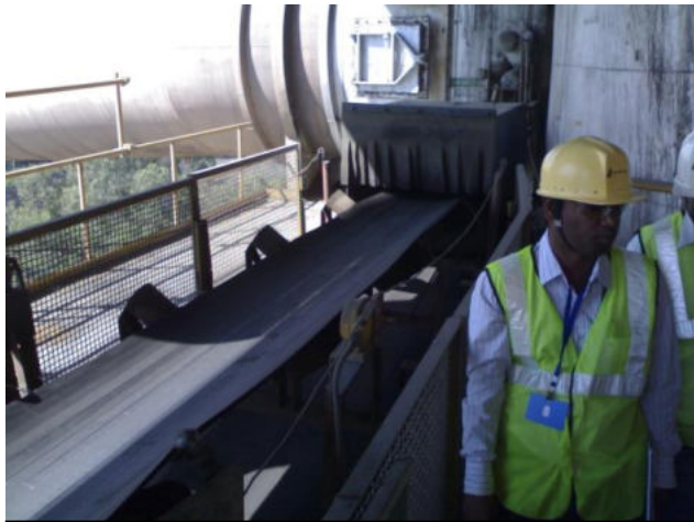
Waste belt conveyor
