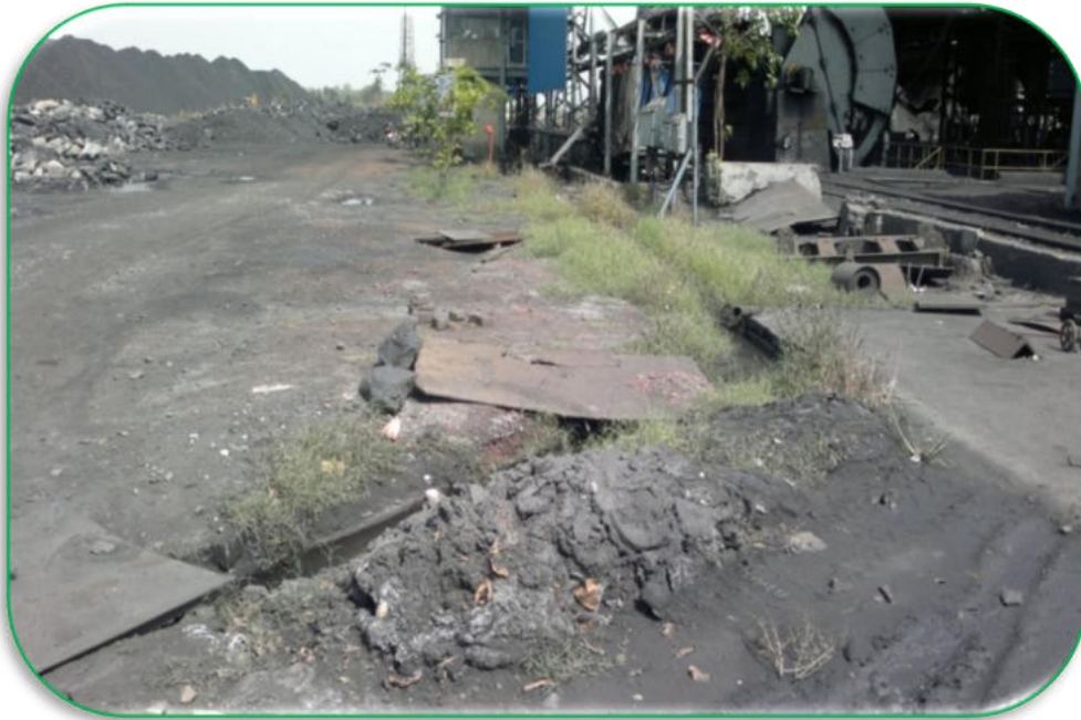
FIGURE 4.15 INADEQUATE WASTE WATER COLLECTION SYSTEM
