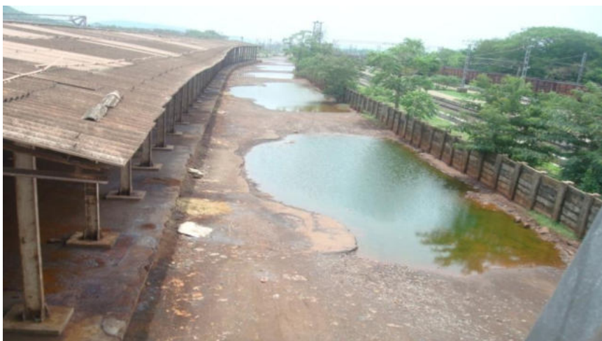
FIGURE 6.5 WATER LOGGING AREA AT SIDING
