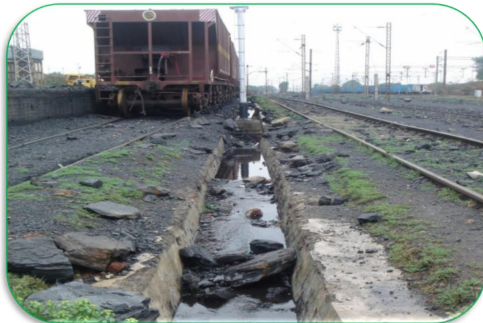
FIGURE 4.16 CHOKED CONDITION OF WASTE WATER COLLECTION SYSTEM
