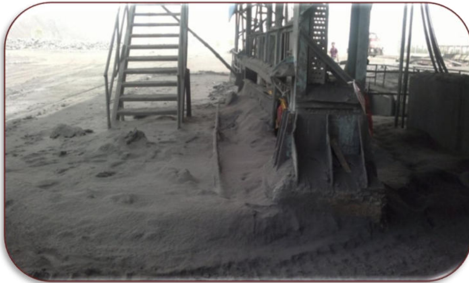
FIGURE 4.6 COAL DUST DEPOSITION AT TIPLING SYSTEM
