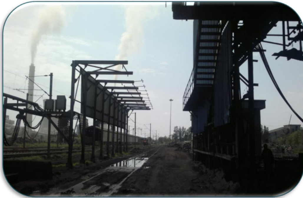
FIGURE 4.12 WATER SPRINKLING SYSTEM
