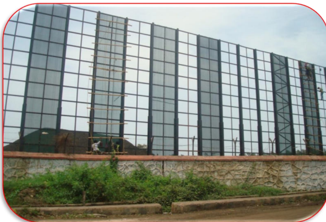
FIGURE 4.14 WIND SCREEN AT PARADIP PORT TRUST
