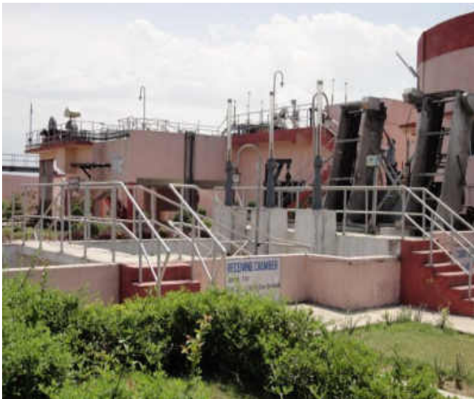
Picture 14: STP at Swarg Ashram
