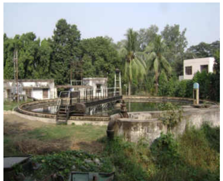
Picture 19: STP at Beur
