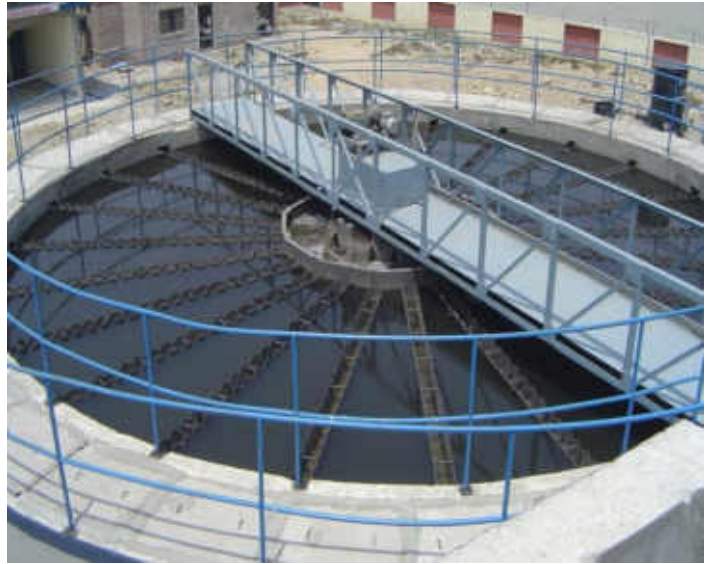
Picture 13: STPs at Srinagar, Uttrakhand
