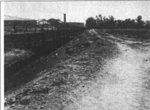
Fig.1: Wastewater accumulation observed at the backside of unit's boundary wall near ETP area
