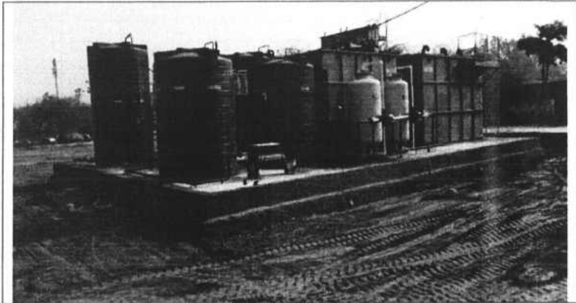
Fig 4a Combined STP of 200 KLD for respondent no 22 & 25
