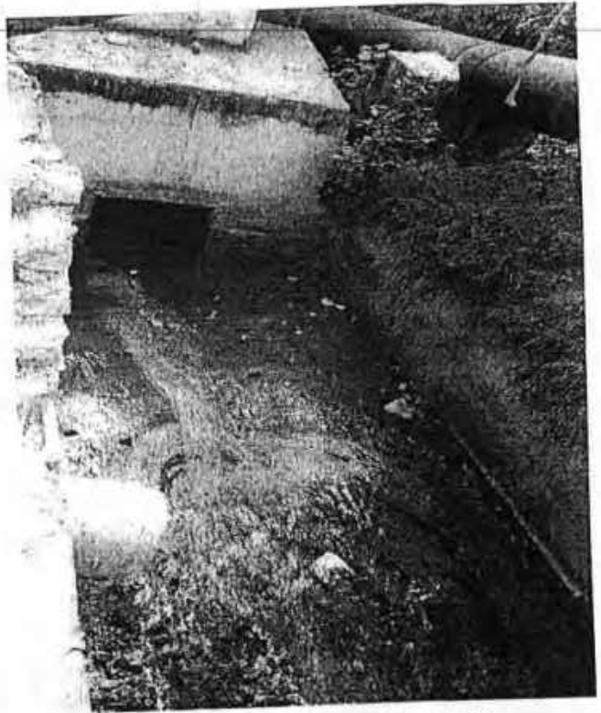
Khyber Pass Drain (Tapped)
