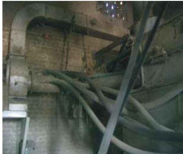
Fig 5.20-Variou suction ducts from milling section to a common cyclone in small rice mills
