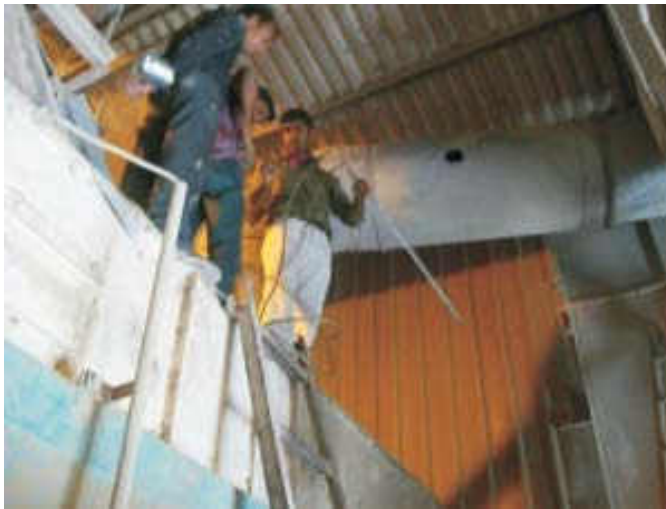
Fig.6.4 Port Hole at Cyclone inlet
