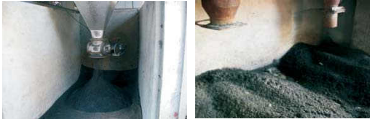
Fig 4.16-A Closed storage of husk fired boiler ash
