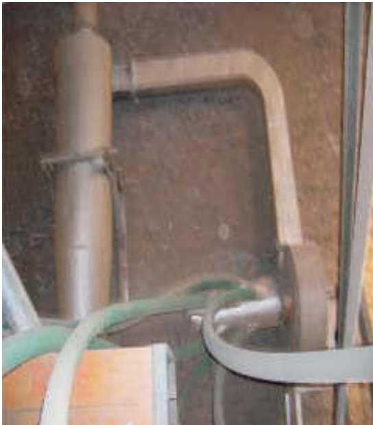
Existing Dust Extraction cum Control System
