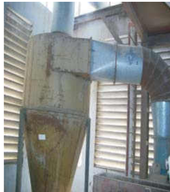
Fig.6.10. Cyclone Inlet (Port Hole 7) on 4 th floor
