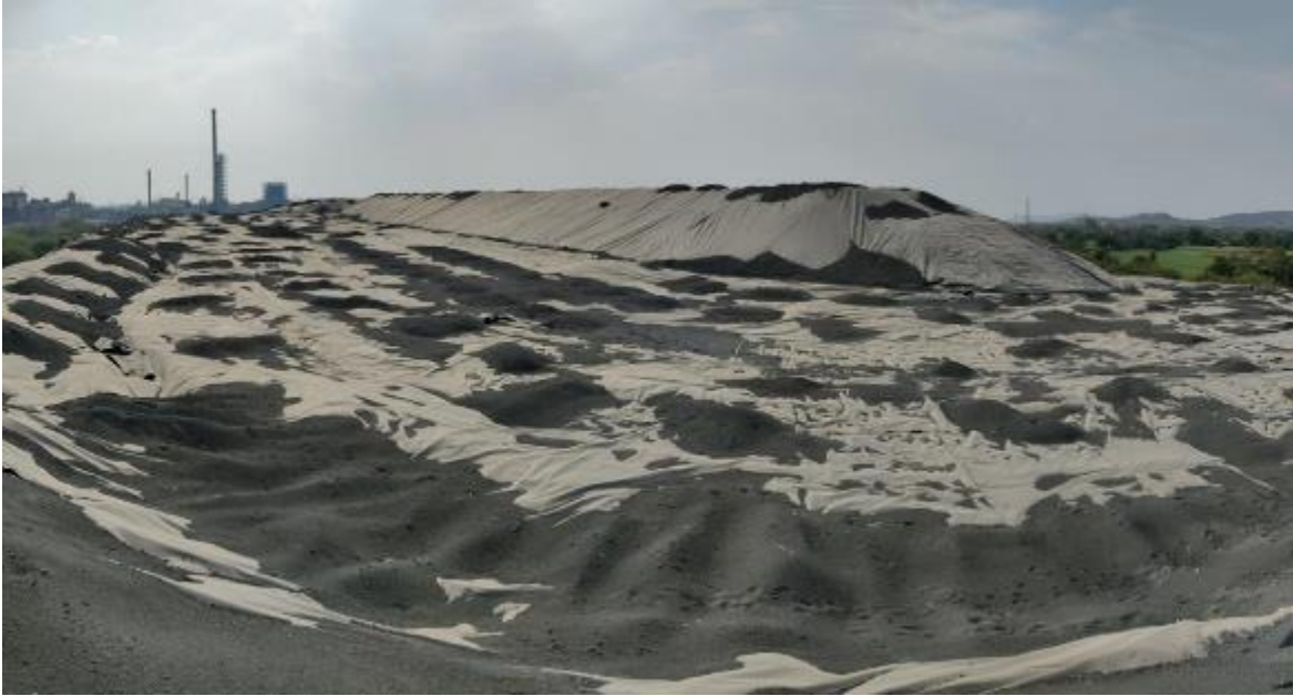
Figure 27: Slag spread over the HDPE sheet to hold it from blowing with the wind
