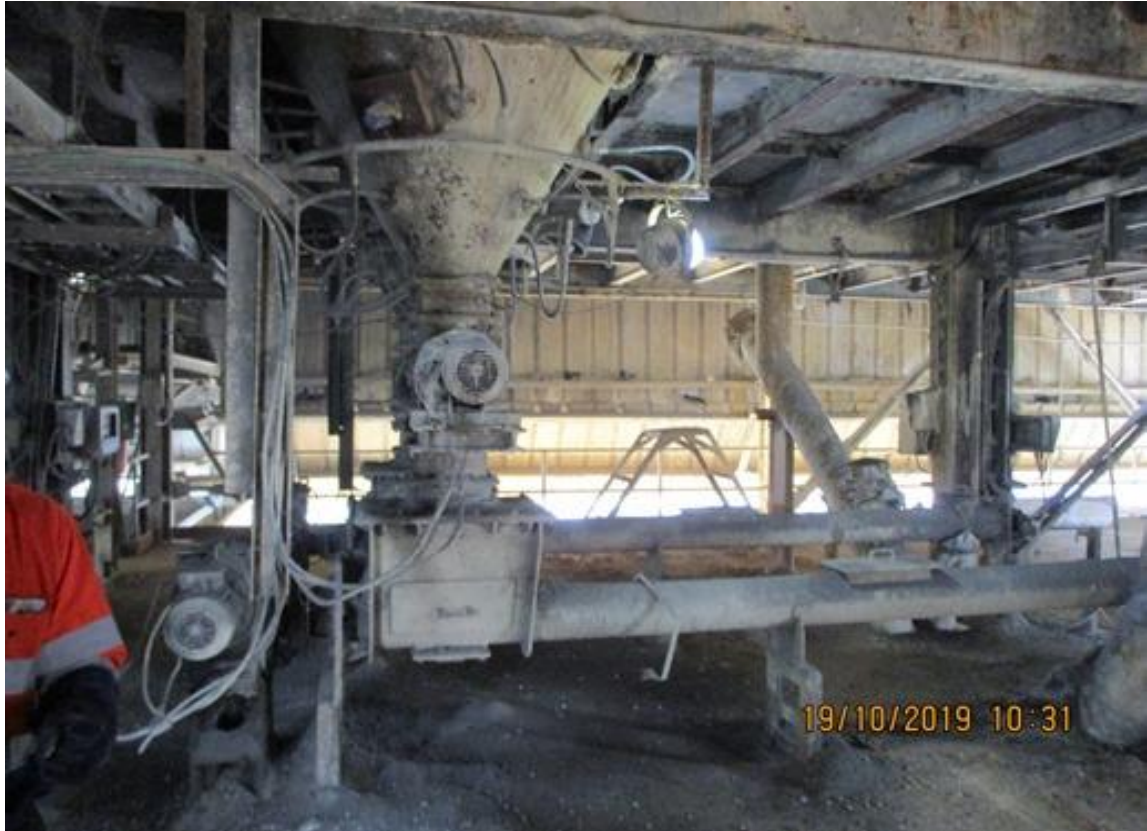
Figure 21: Lime Feeder System at Chanderiya hydro smelter
