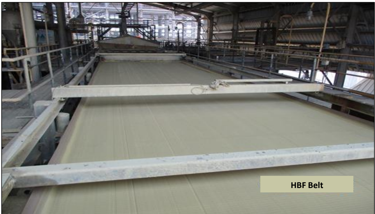
Figure 22: Horizontal Belt Filter
