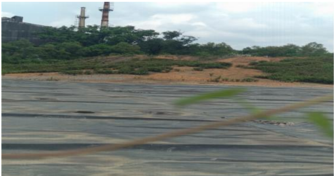
Figure 14: Stabilized Jarosite yard at Edayar Zinc Ltd. showing HDPE lining and stock
