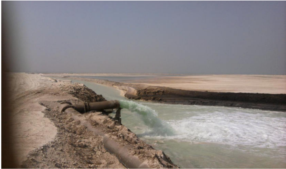
FIG. 8. Pumping of phosphogypsum to the 'Ridge Dyke' in the form of slurry to the phosphogypsum stack
