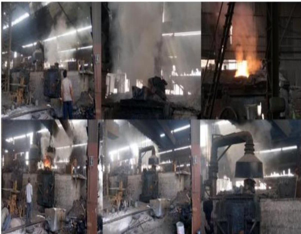
Figure 35: Existing Induction Furnace in a Factory over IGP
