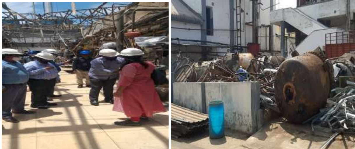
Photo taken during inspection of Production exploded reactor 504 kept in unit premises block-5
