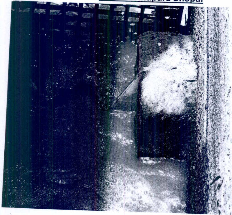
Inlet V-Notch at CETP inlet
