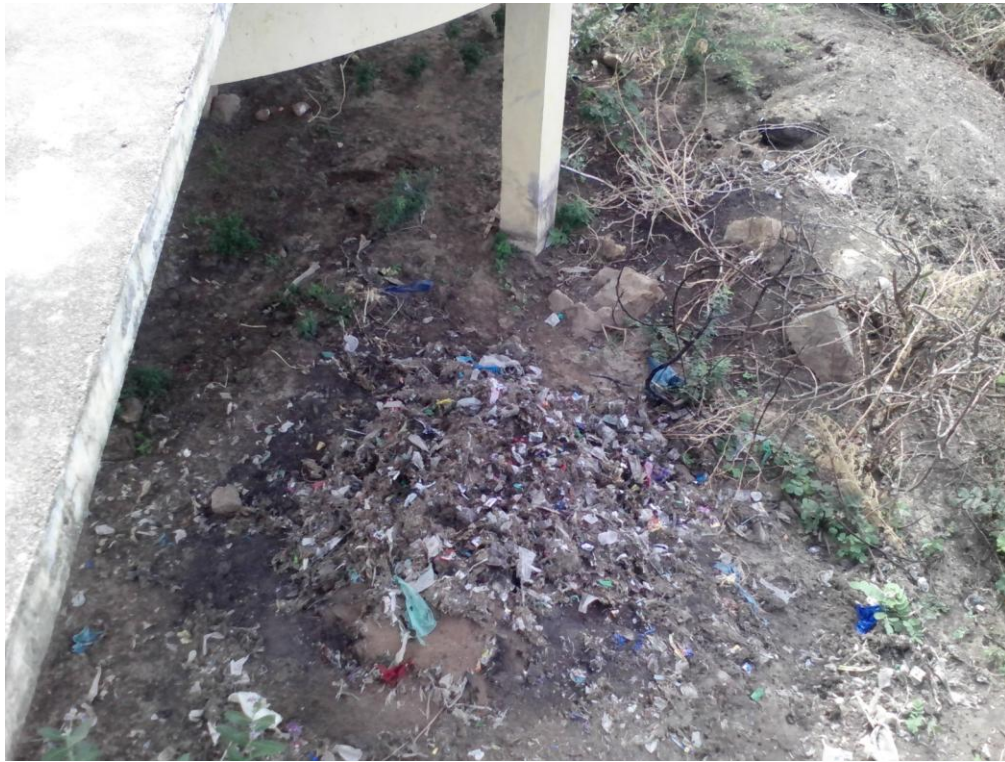
Fig 4: Solid waste from screen chamber is removed and dumped inside the unit creating unaesthetic condition.
