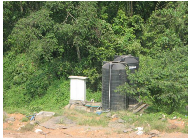
Fig.2: Leachate Storage tank (Sintex) with pumping arrangement.
