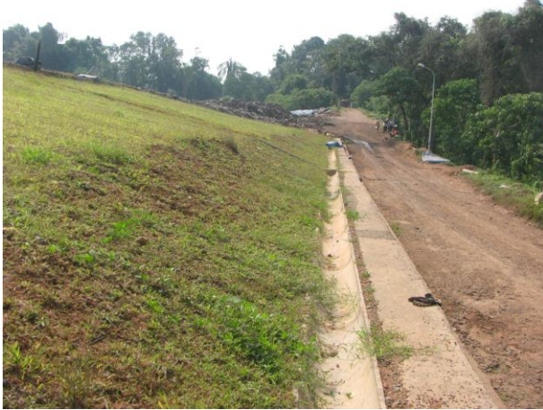
Fig.7: Cells cover bottom is provided with garland drain. The internal roads are not paved.
