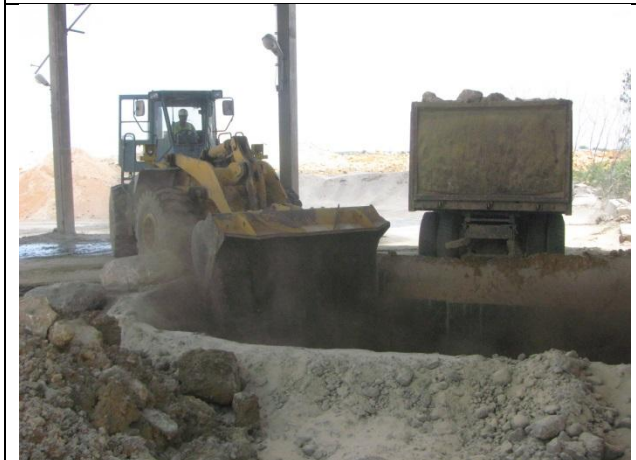
Fig.3: ETP sludge charging along with lime stone to the crusher
