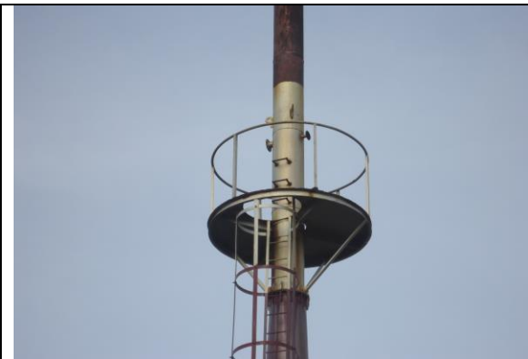
Fig. No.2 Platform Condition
