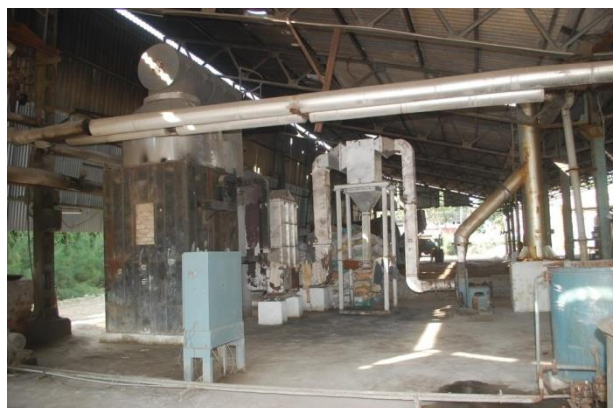
Plate 8. Thermic Fluid Boiler and its APCs
