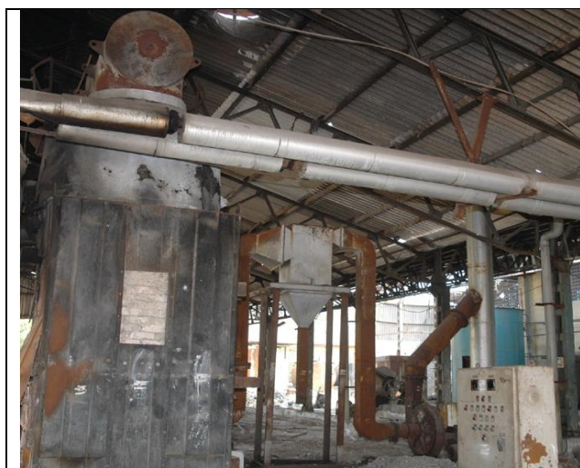
Fig.7. Air Pollution Control System in Thermic Fluid 2T/Hr Boiler during First Monitoring
