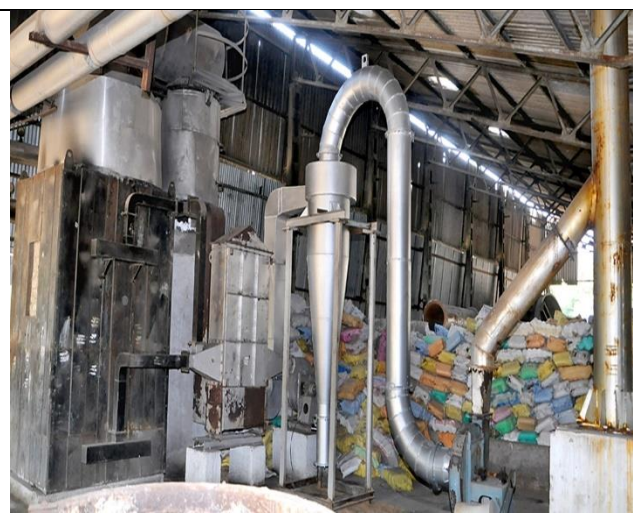
Fig.8. Air Pollution Control System in Thermic Fluid 2T/Hr Boiler during Third Monitoring
