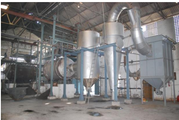
Plate:9 Enhanced Air Pollution Control Devices installed
