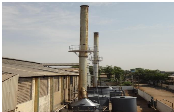
Plate:10 Stack Connected with Rotary Furnaces
