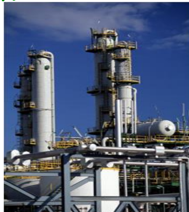
Flue Gas Desulfurization System
