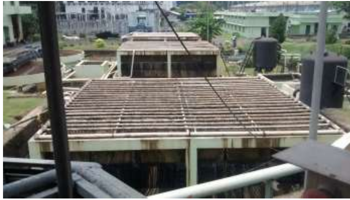
Non-operational Bio Towers
