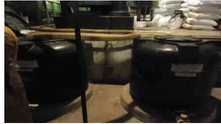
Fig 16: Concentrated effluent storage tanks
