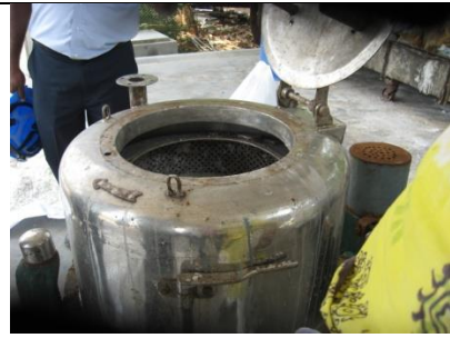
Fig 21: Centrifuge to recover sodium sulphate salt
