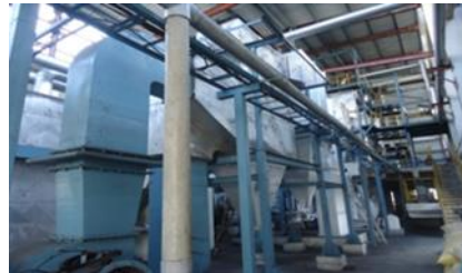
Fig 33: Arrangements made for Burning of odours gases in boiler
