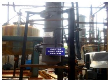
Fig. 42 : Carbon bed for Ejector sump
