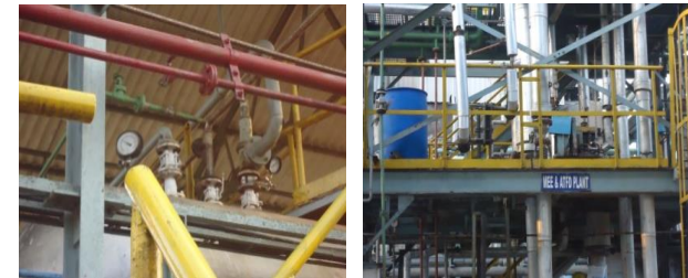
Fig 55: Rupture Disc Fig 56: MEE & ATFD Provided to Acetaldehyde tank
