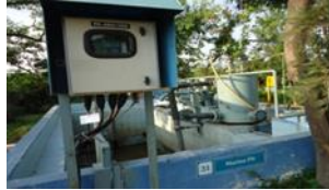
Fig 5: pH on line meter
