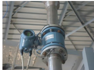
Fig 60: EMFM installed to quantify the RO reject feed to MEE
