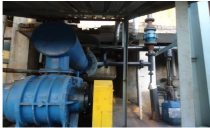
Fig53: Vents connected blower
