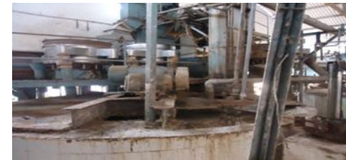
Fig 34: Anti odour spray system installed at Bones washing section
