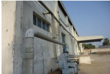
Fig 32: Blower to suck the odourous air from the godown UASB
