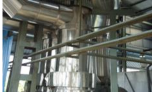
Fig 4: Wet scrubber to avoid acidic vapour
