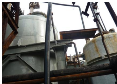
Fig. 41: HCl and SO 2 Scrubber
