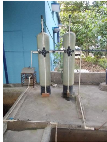
Fig.14: Sand filter and activated carbon filter installation at ETP.
