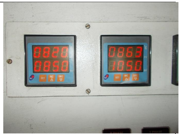
Fig.2: Operating parameter indicator, Secondary temperature showing only 863°C against 1050°C.
