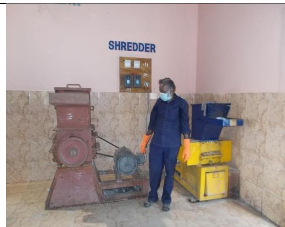
Fig.16: shredder installed and found in operation.
