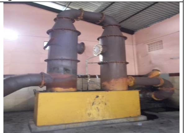
Fig.4: Scrubber connected to 100 kg/hr. incinerator & No mist collector attached
