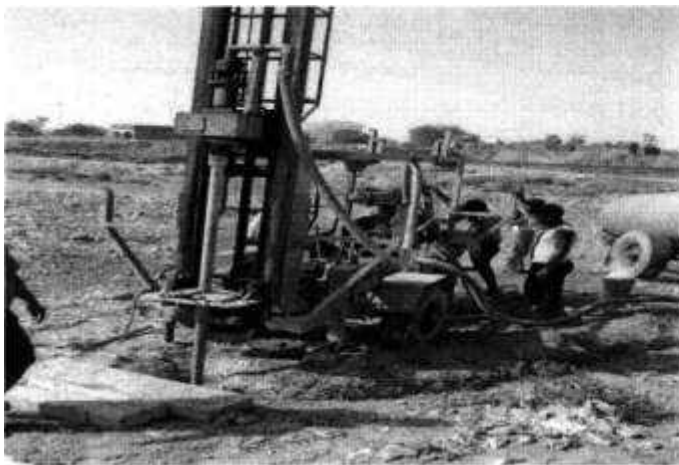
Step iii): Mode of drilling using Direct Circulation System Rotary (Mud Rotary Drilling) method
