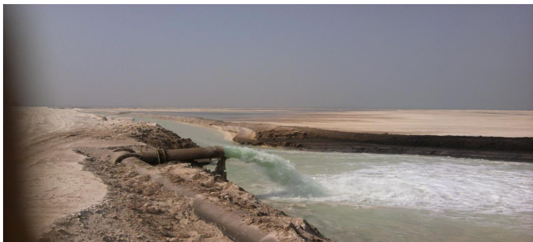
Figure 9: Pumping of phosphogypsum in the form of slurry to the 'Ridge Dike' of the phosphogypsum stack
