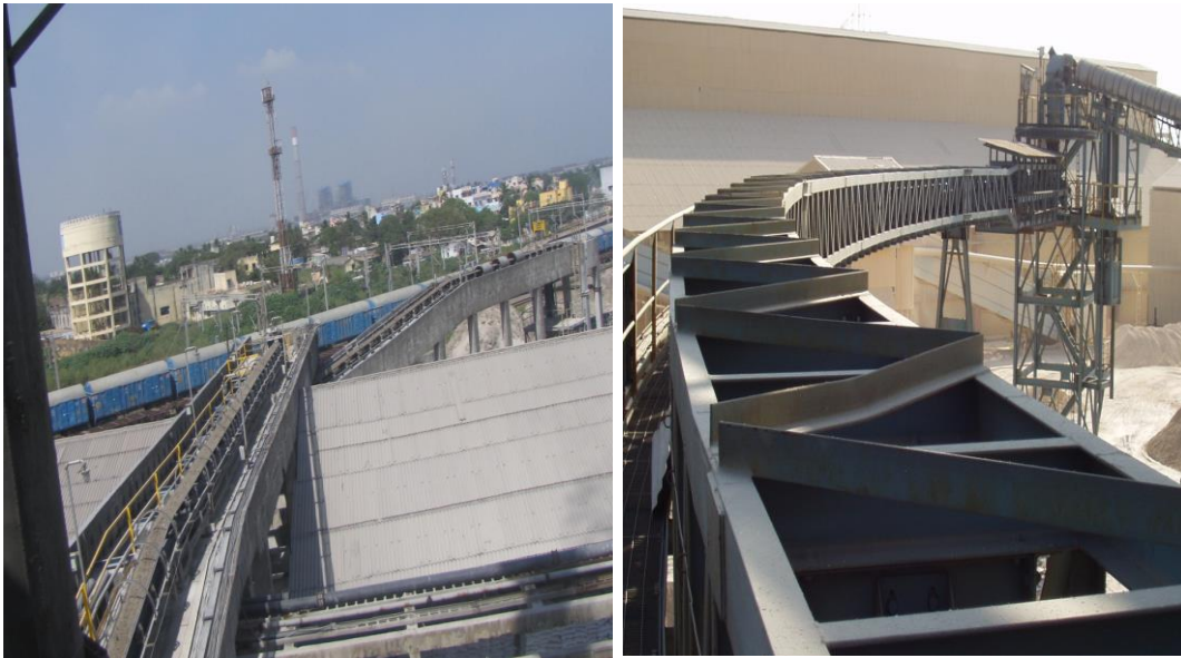
Figure 4 & 5: Conveyance of phosphogypsum to the stack area by 'Belt Conveyor'
