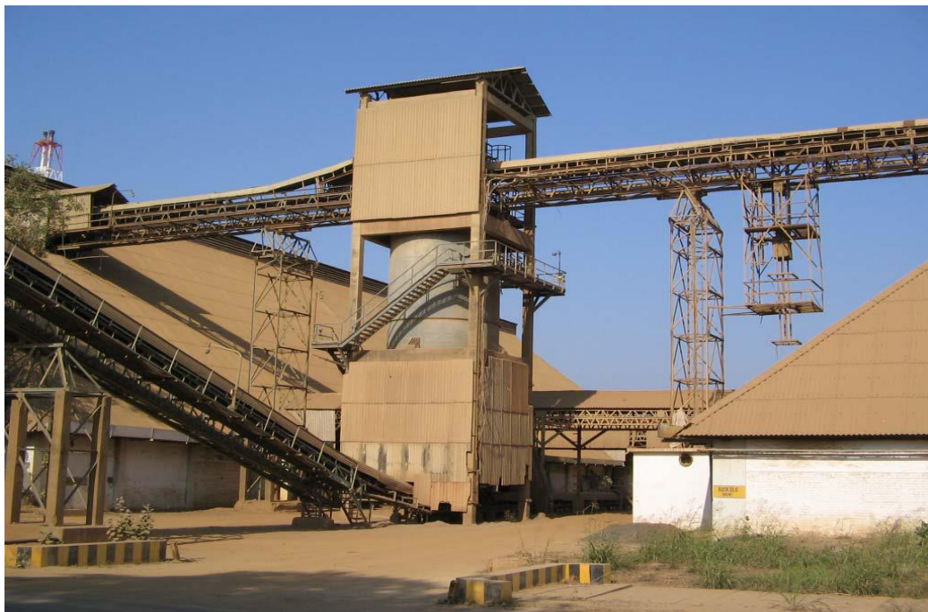
Figure 2: Phosphate rock silo & conveyance system
