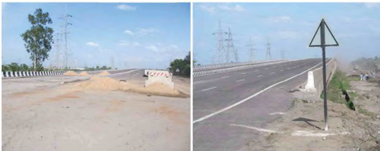
Fig-5.1 Construction of flyover in the highway in front of M/s BSL
