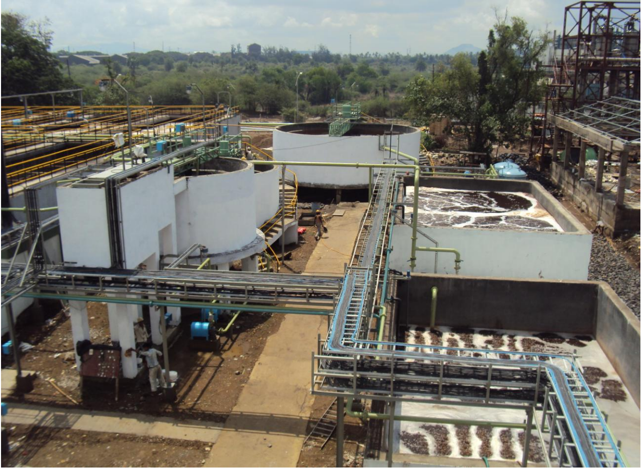
Aerial view of Full fledged ETP under operation by one of bulk drug industry from Tarapur
