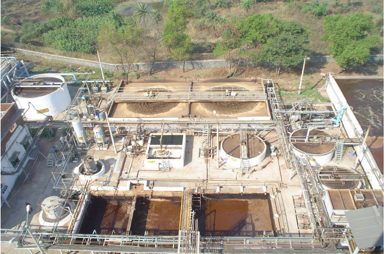
Aerial view of Full fledged ETP under operation by one of bulk drug industry from Tarapur
