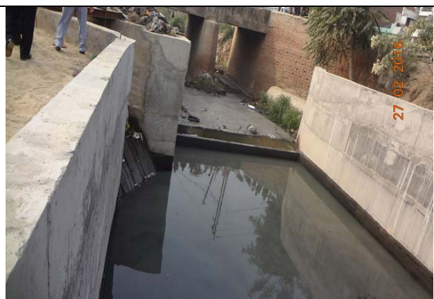
Photo 8: Conveyance system for Bingawa STP
