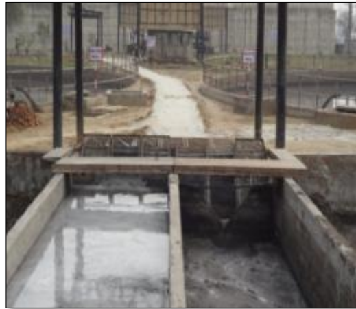
Tannery Wastewater Inlet to CETP
