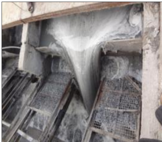
V – Notch for measurement of Effluent
