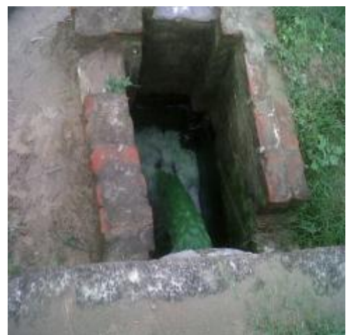
Photograph-Outlet of STP
