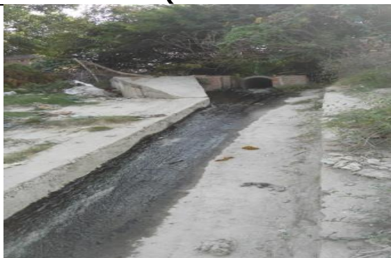
Fig- Sampling point of Jail Drain
