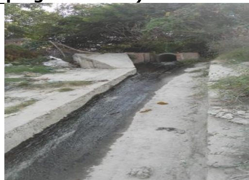
Fig-Confluence point of Jail Drain & River Ganga
