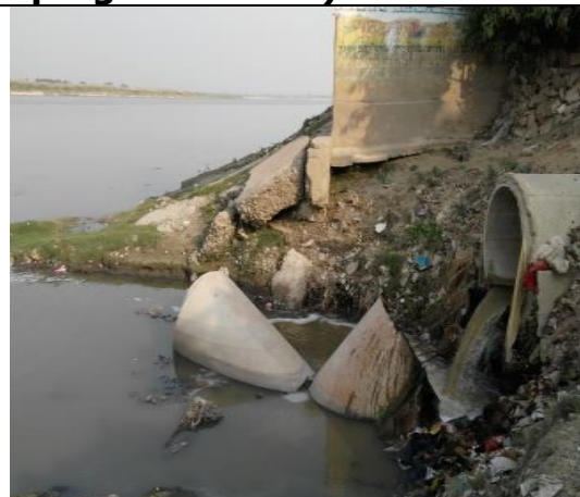
Fig- Confluent point of Tefco Drain & River Ganga
