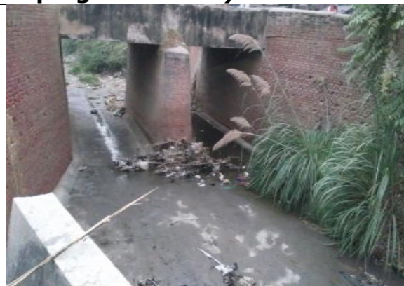
Fig-COD Nala Tapped into STP
