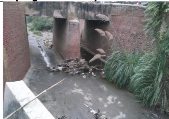
Fig-COD Nala Tapped into STP
