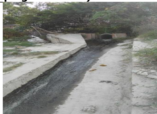
Fig-Confluence point of Jail Drain & River Ganga
