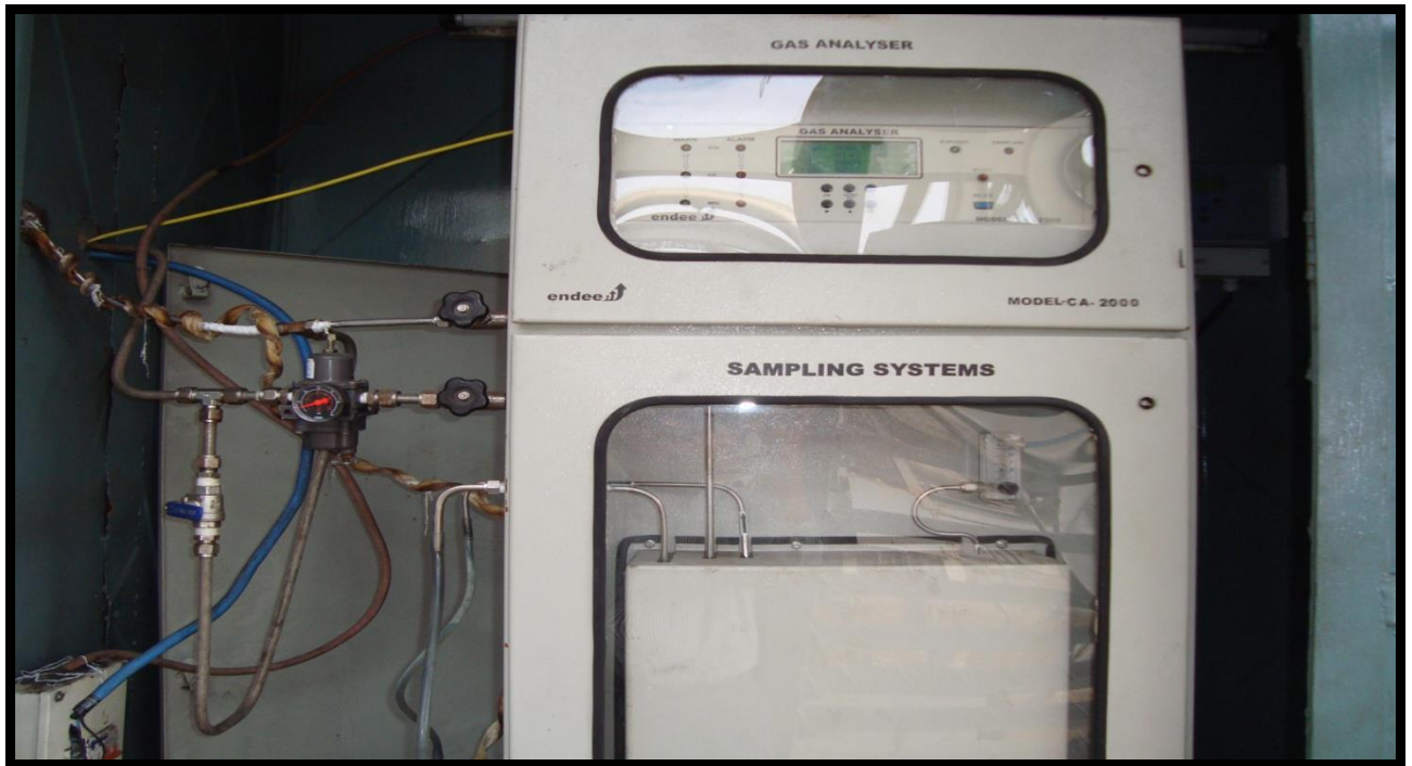
BOILER STACK CONTINUOUS MONITORING SYSTEM AT MPL Plant-I
