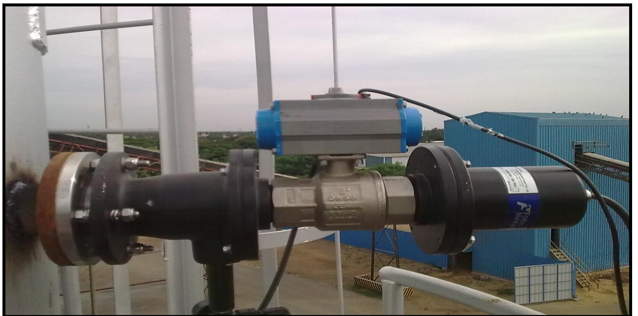
Stack Emission Monitoring online at M/s SRF Polymers
