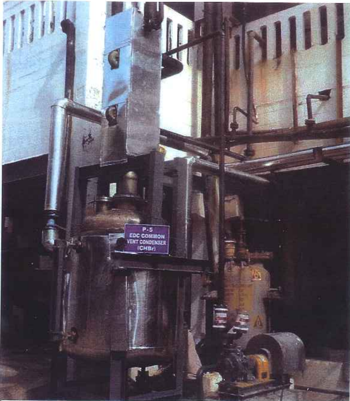
Tagros Chemicals India Limited - Cuddalore Common Vent Chiller Common vent chiller with -20C chilled brine circulation for VOC reduction from plant vents
