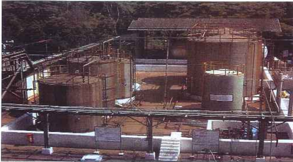
Formaldehyde Storage tank Farm
