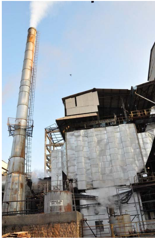
ESP and Chimney provided to Chemical Recovery Boiler of MPM
