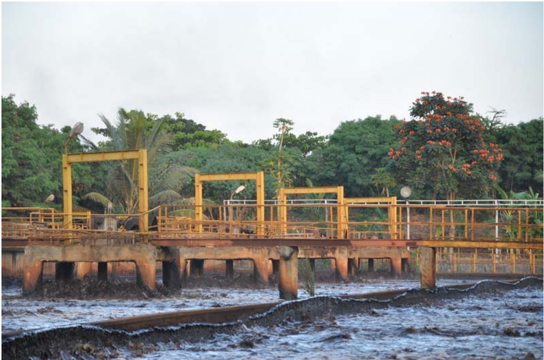
Aeration tank of MPM
