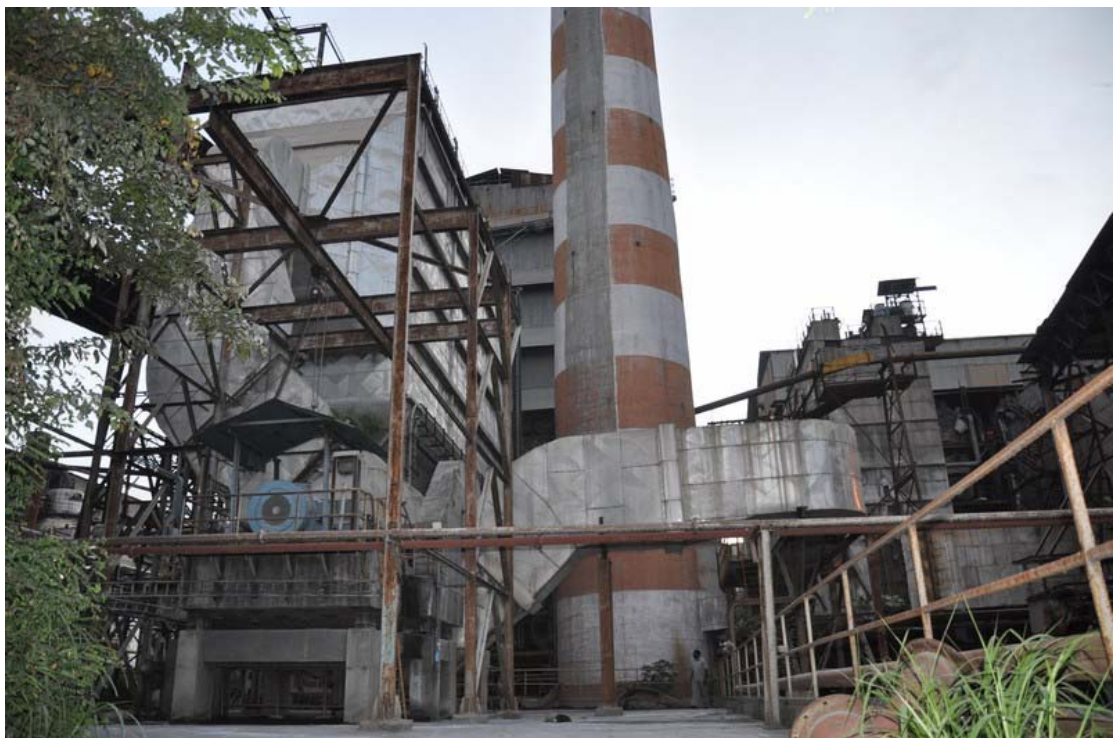
ESP and common Chimney provided to Coal fired Boilers of MPM
