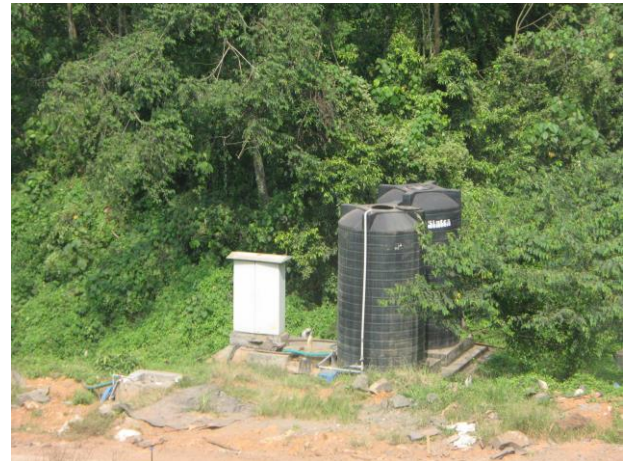
Fig.2: Leachate Storage tank (Sintex) with pumping arrangement.
