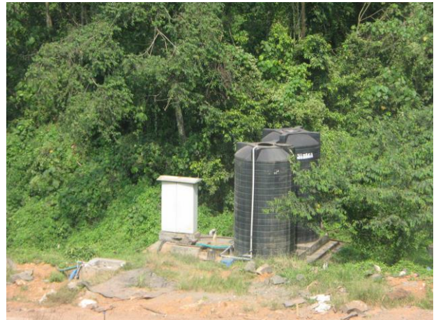
Fig.2: Leachate Storage tank (Sintex) with pumping arrangement.
