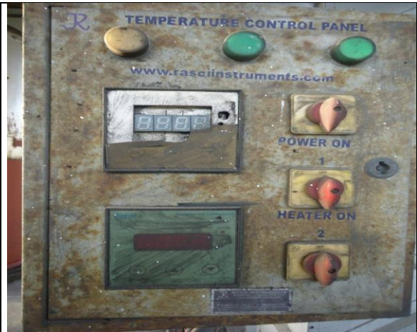
Fig No.1 Temperature Display not working
