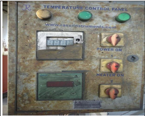
Fig No.1 Temperature Display not working
