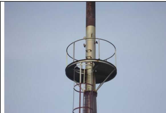
Fig. No.2 Platform Condition
