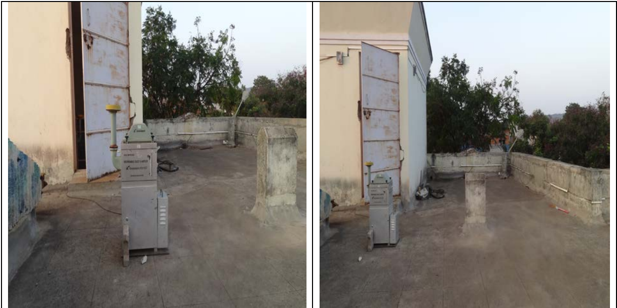
RDS is placed near to the entrance wall
